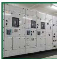
LV distribution panels for motor controllers, small power, & lighting DBS
