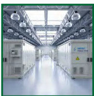
UPS input & output distribution panels for parallel redundant UPS systems
